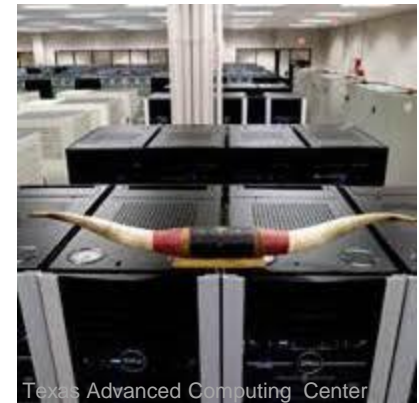
Texas Advanced Computing Center Longhorn system at TACC
